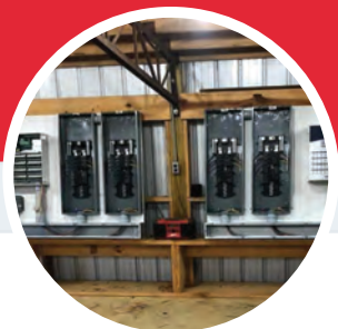
CONTROLLER SYSTEM DESIGN & INSTALL
